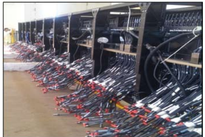
Figure 12. RF Cables in the AAAU.
