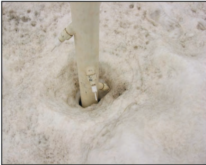
Figure 6. Void that developed around the central column.
