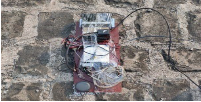
Figure 11. GNSS receiver, radio and battery mounted on a single plate.
