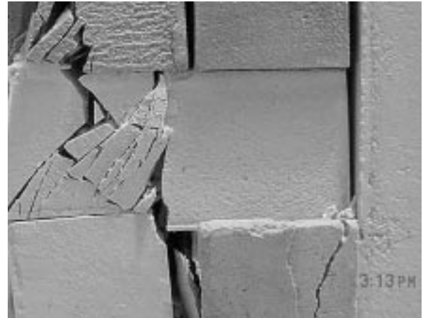
Figure 7. Shearing fracture passing through a series of tensile cracks.
